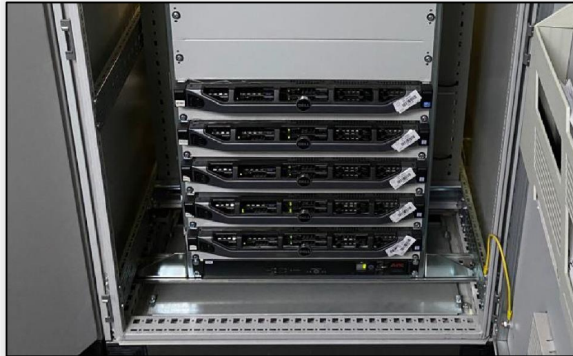
Figure 4.16: Dell PowerEdge R420 rack servers.
