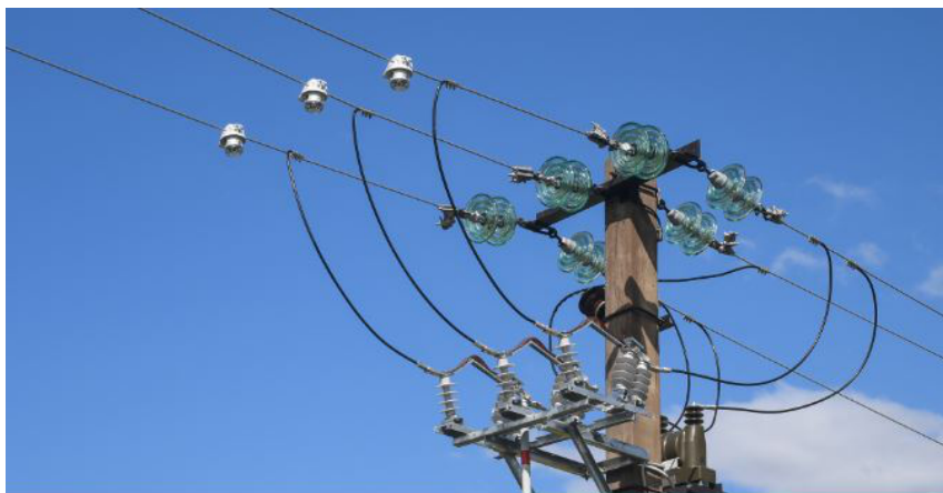
Figure 2. Medium voltage overhead line Fault passage indicators [3]
