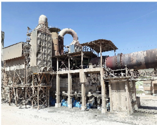
(a) pre-heater tower at the right along with rotary kiln laying in horizontal to the left.
