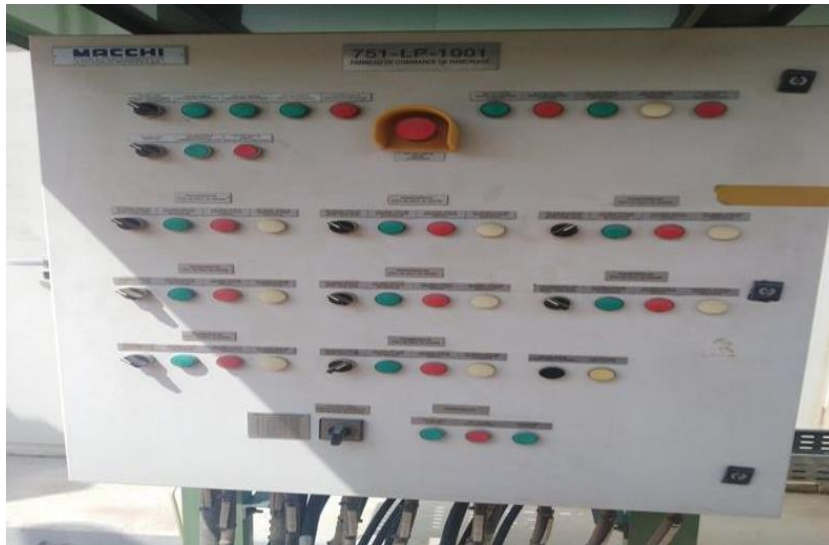
Figure 3.6: Sootblowers local panel.
