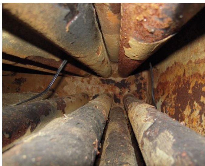
Figure 3.1: The accumulation of soot on boiler tubes.
