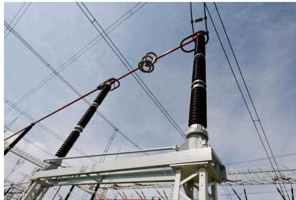
Figure 1.11: High voltage isolating switch.
