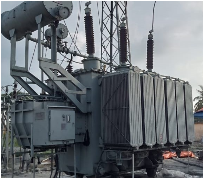
Figure 1.8: Power Transformer 220kV/60kV.
