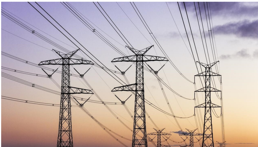
Figure 1.18: Overhead transmission lines.
