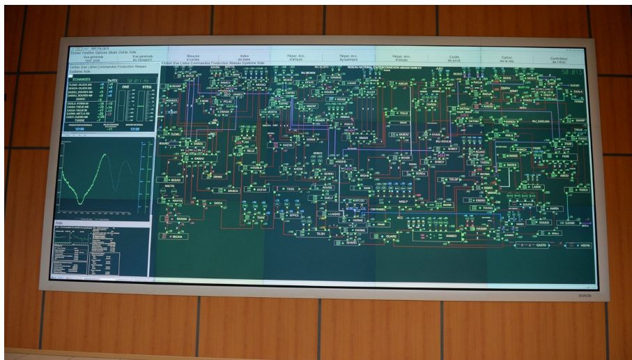
Figure 2.2: Control center of dispatching.
