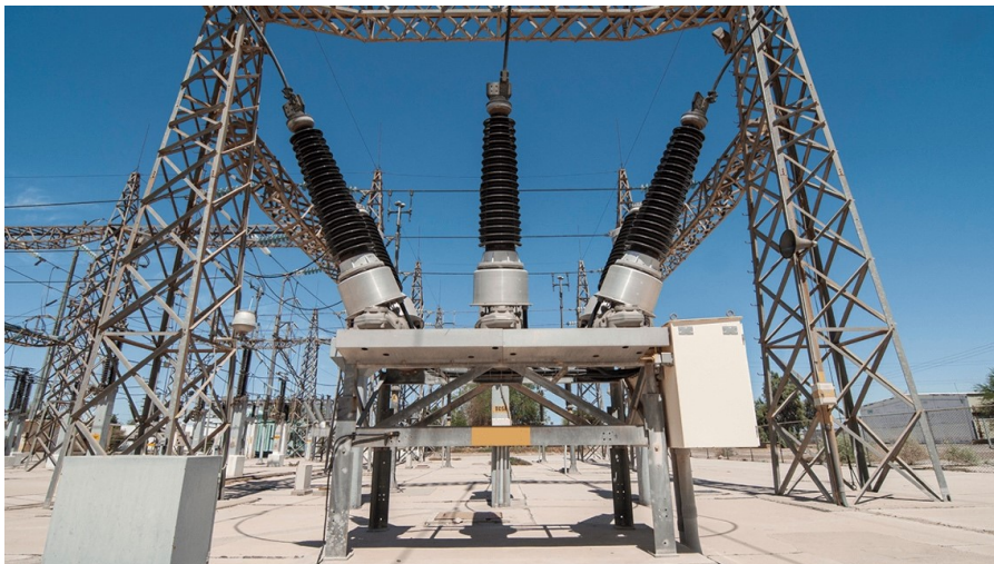
Figure 1.9: Sulfur Hexafluoride (SF 6 ) Circuit Breakers.
