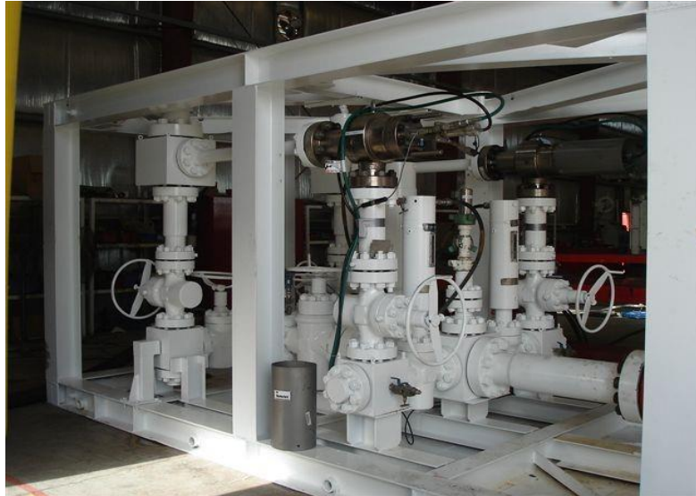
Figure III. 18: MPD Choke-Semi Automated (Weatherford, 2008)
