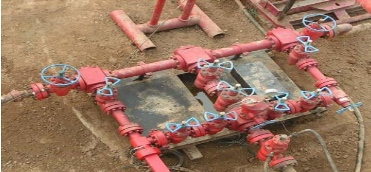
Figure III.21 : UBD Choke Manifold
