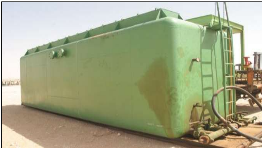
Figure VI.05: Bac de stockage
