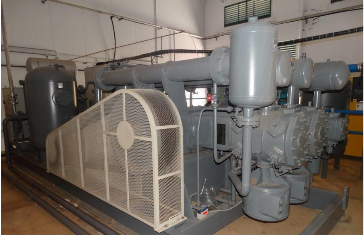
Figure II.5 Compresseur (ABC 4HA-6-TER-LT)
