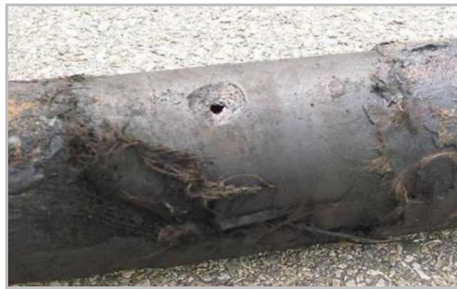
Figure II.7. Corrosion externe (Sainson, 2007).
