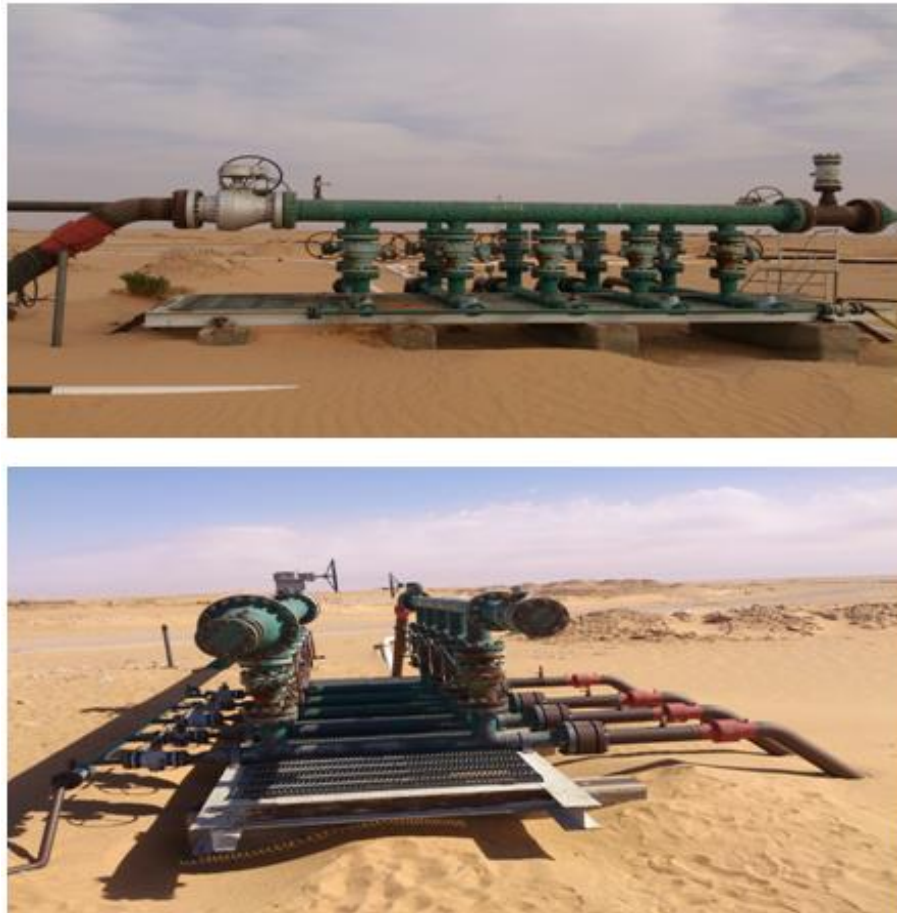
Figure III.8: Manifold de production [1]
