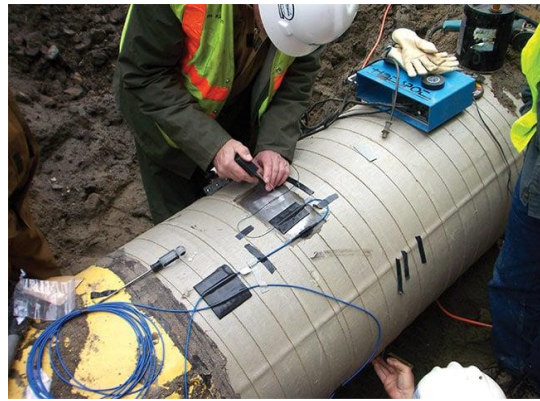
Figure 1. 7: optical fiber sensor installed on an actual pipeline
