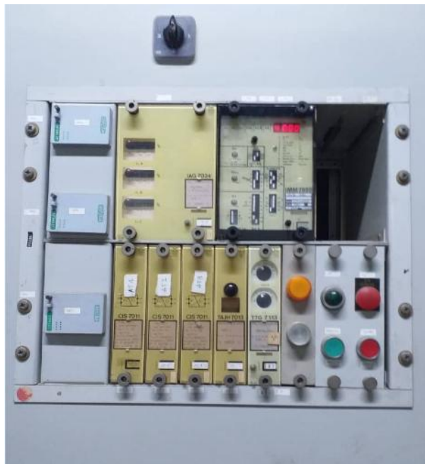
Figure III. 9: Les relais de protection (motopompe eau de mer)
