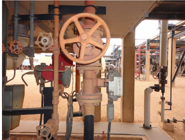
Figure II. 14 : La vanne HV109.
