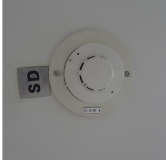
Figure III. 8 : Simplex 4089-9714 Smoke Detector [31]
