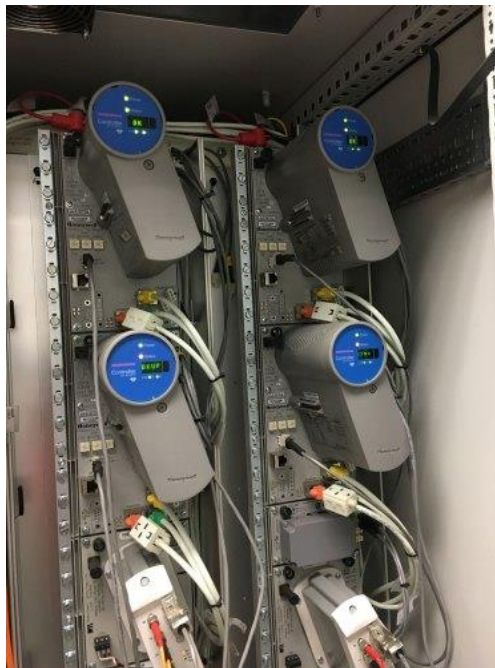
Figure IV. 33 : Honeywell EPKS Controllers
