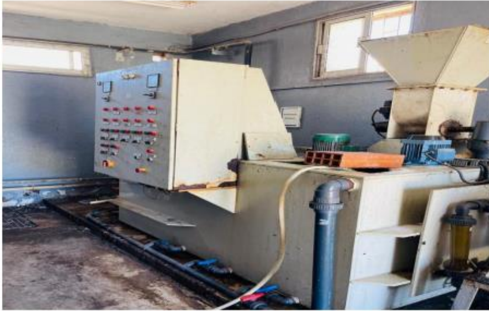
Figure.I.23: Polymer preparation station.
