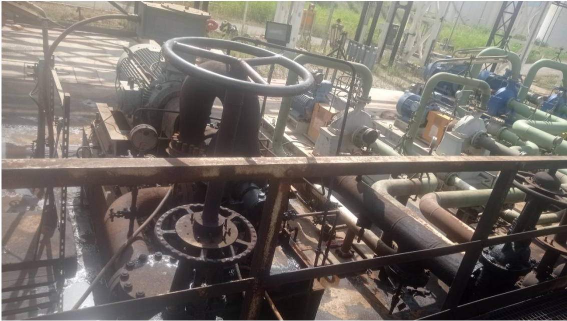
Figure II.13: installation de pompe G111
